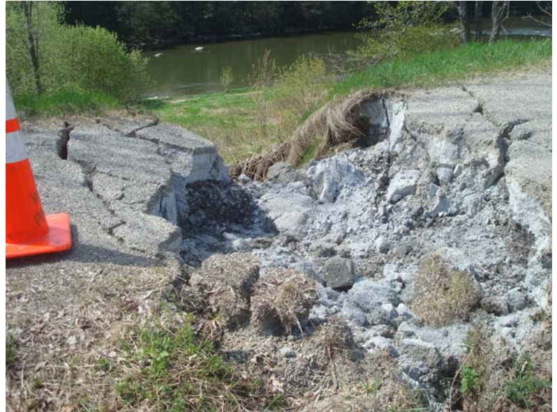
A failed culvert beneath the MVRT closed the Trail for a couple of weeks in May
